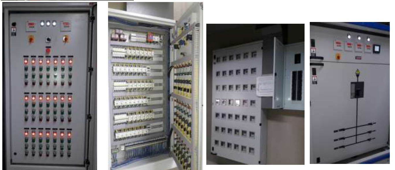
Automatic Lighting Control by timer setting
